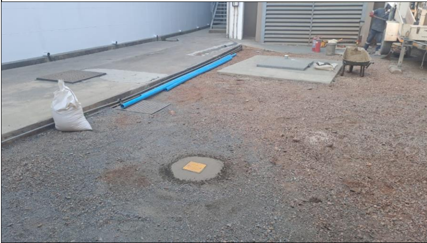
Photograph 3: Typical completed monitoring well and headworks.
