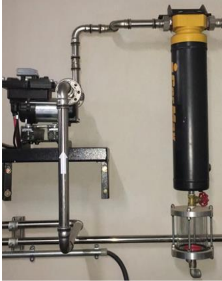
Figure 4: Typical filter system for Day tanks
